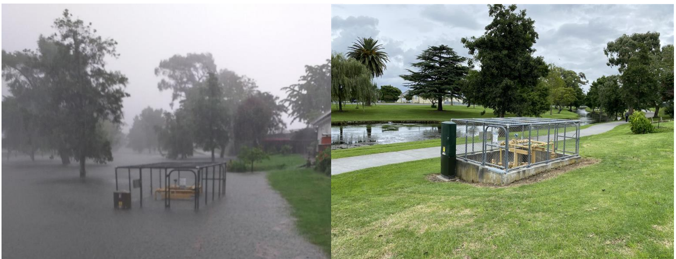
Figure 4: Georges Drive DRS during the 2021 floods, left, and the green raised SCADA cabinet after remediation in 2022. Note, the green cabinet reaches the ceiling of the enclosure in the second photo.
